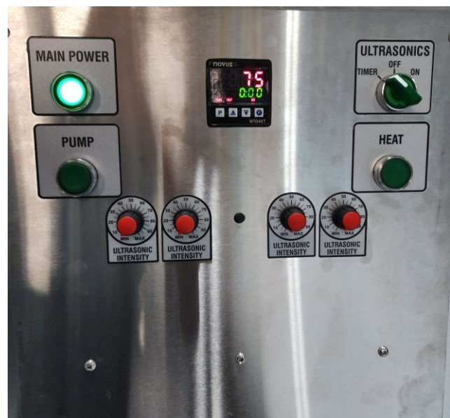
Figure 16: Generator Timer Cycle Done
