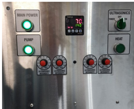
Figure 21 Pump Manual Control On
