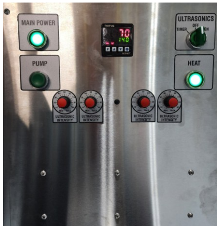
Figure 22: System Control On
