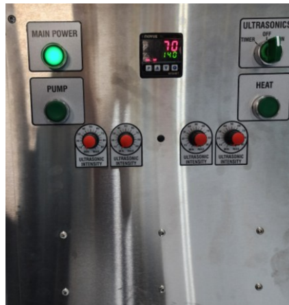
Figure 23: System Power On
