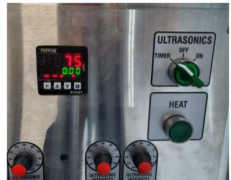
Figure 14: Generator Timer Cycle Done
