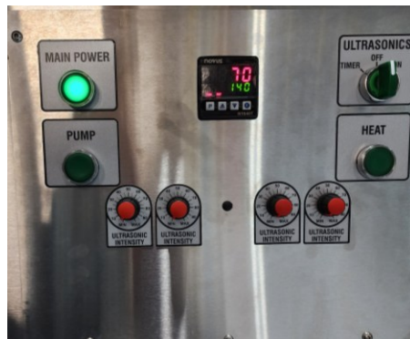
Figure 20 Pump Manual Control Off
