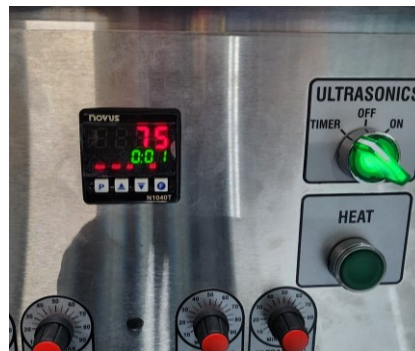
Figure 13: Generator Timer Running
